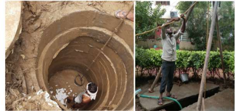
RWH Cleaning at MCG Sector 22 and 23 through Manual Labour and Bockey Machine
