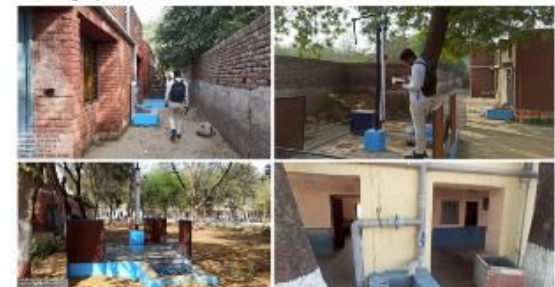
RWH structures at Govt Schools
