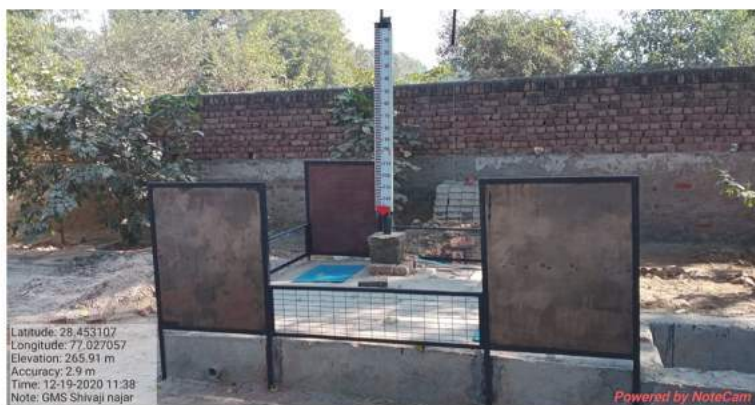
Rainwater Harvesting Structure at Govt. Middle School, Shivaji Nagar, Gurugram
